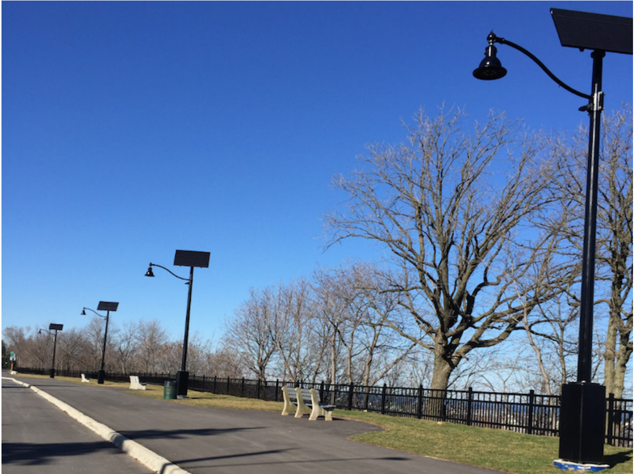
Illumient Smart Off-Grid Lighting along Mountain Brow Blvd, City of Hamilton.
